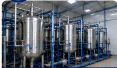
Sistem Filtrasi & Water Treatment
